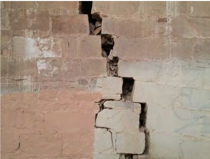
PHOTOGRAPH 7: East wall cracking
