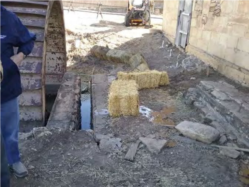
PHOTOGRAPH 21: Straw bales to catch surface runoff
