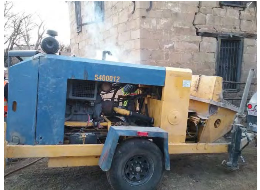
PHOTOGRAPH 12: Grout mixer and pump
