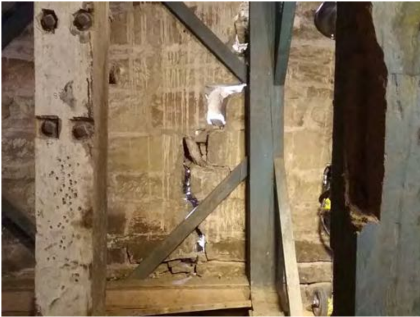
PHOTOGRAPH 15: East wall crack inside building
