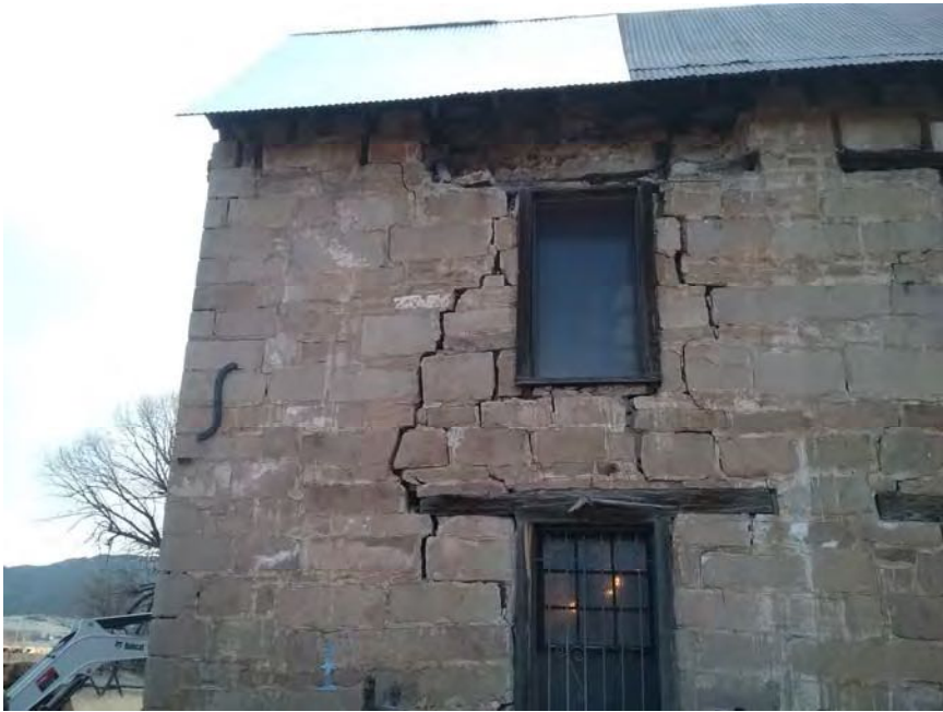
PHOTOGRAPH 3: West wall cracking
