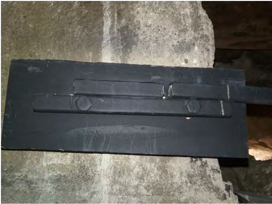
PHOTOGRAPH 31: Movement monitoring gauge at E. wall crack
