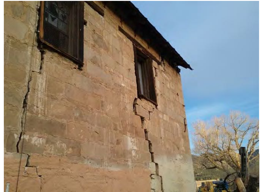
PHOTOGRAPH 6: East wall cracking
