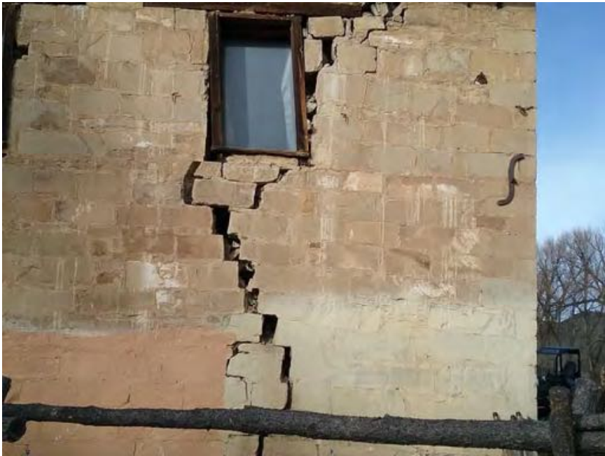
PHOTOGRAPH 17: East wall crack at 2nd story window
